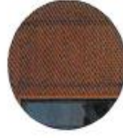
EXPOSED BARE CORTEL STEEL
